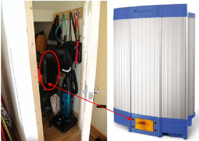
Figure 4. PV converter as installed in LILAC houses and catalogue image.
