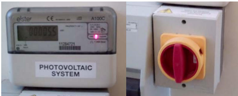
Figure 5. PV meter and switch installed in LILAC (photo MBN).
