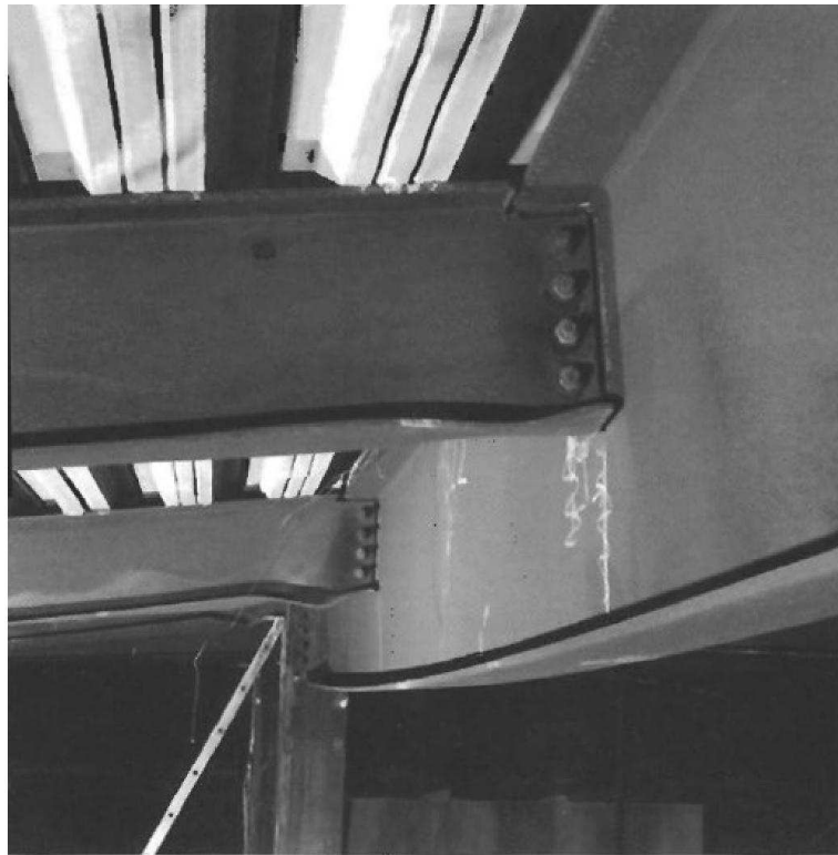
Figure 3. Fin-plate connections of secondary beams showing local buckling [21].
