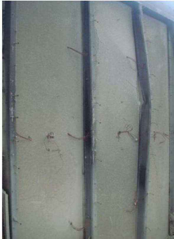
Figure 4. Cold-formed steel frame after fire [12].
