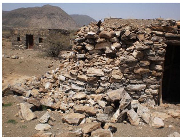
Fig. 5 Building damaged by the 31 March 2011 earthquake. Better constructed walls, as seen in the background, sustained only cracking
