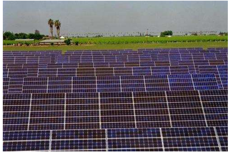
A solar plant in Fresno, CA. Source: www.nrel.gov
