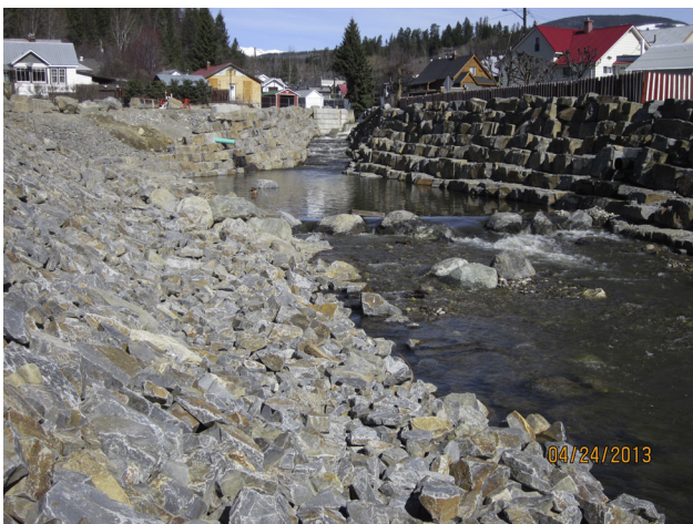
Fig. 6. Photo of the first phase of work on the Mark Creek Flume Flood Management and Stream Rehabilitation Project in April 2013 (photo: T. Pollock, 2013).
