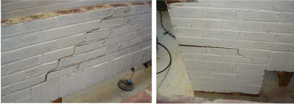
Fig. 5 Failure mode of the masonry wall panel as observed from the experiment
