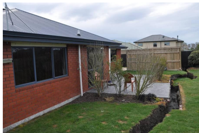
Figure 5.20: Ground failure feature extending through the backyard of a home on the south side of Courtenay Drive in the South Kaiapoi residential community.
