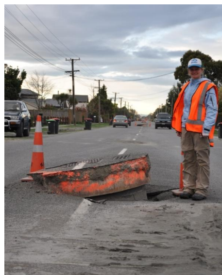
Figure 7.47: Uplifted manholes along Lower Styx Road, note the continuation of pattern in the foreground (43.4113°S, 172.6930°E).
