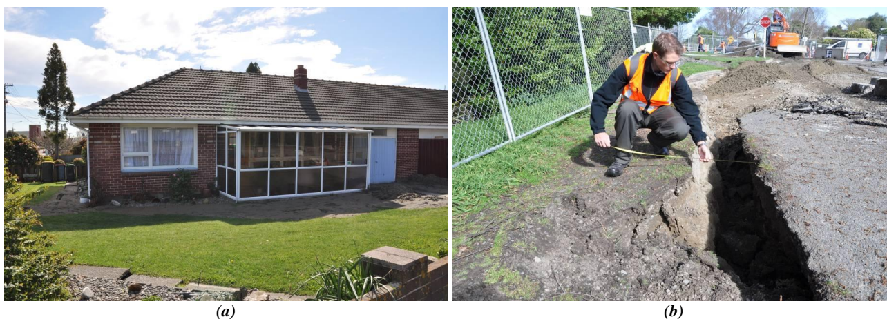
Figure 5.25: (a) Rigid body rotation of a residence in Dallington (Locksley Avenue) due to liquefaction and (b) lateral spread features directly fronting the home. Surveys of ground features at this location are associated with T7 (refer to Figure 5.27).
