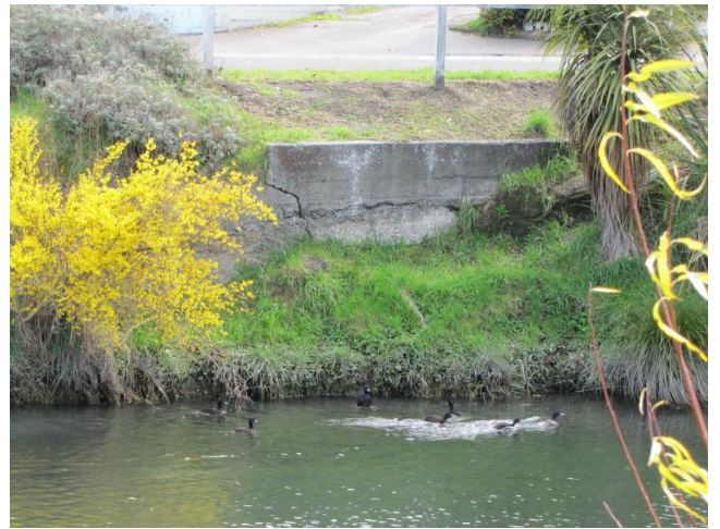
Figure 7.15: Cracking of retaining wall, north bank of the Avon River.
