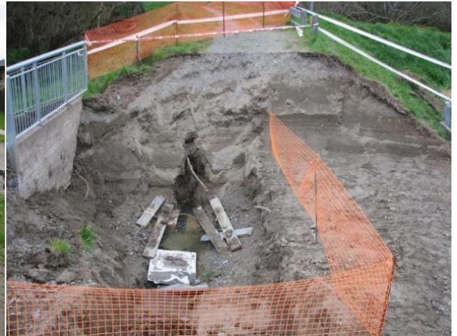
Figure 6.26: Photo 28: Failed drainage conduits running underneath the stopbank on the south side of the Kaiapoi River. The location of this photograph is denoted in Figure 6.2. (43.388679°S, 172.666203°E).
