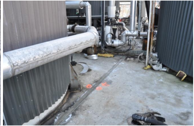
Figure 7.44: Repair of lateral spread cracks within the Fulton Hogan Bitumen Plant, nearby Tank 3. (43.6085°S, 172.7150°E).
