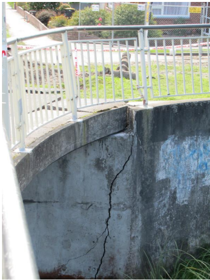
Figure 7.14: Cracking of north abutment, Swanns Road Bridge.
