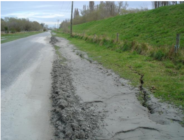
Figure 6.5: Photo 2: Crack running along base of stopbank on Coutts Island Rd (landside) and liquefaction ejecta. (43.424466°S, 172.629907°E).
