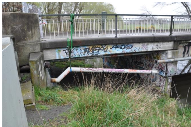
Figure 7.31: Damage to sewage pipe at the Kainga Road Bridge (43.3997°S, 172.6916°E).
