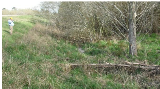
Figure 6.6: Photo 3: Liquefaction ejecta (centre of photo) along the base of the stopbank on Coutts Island Rd (riverside). (43.424093°S, 172.630468°E).
