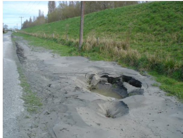
Figure 6.4: Photo 1: Large sand boil at the base of the landside of the stopbank on Coutts Island Rd. (43.425018°S, 172.628442°E).
