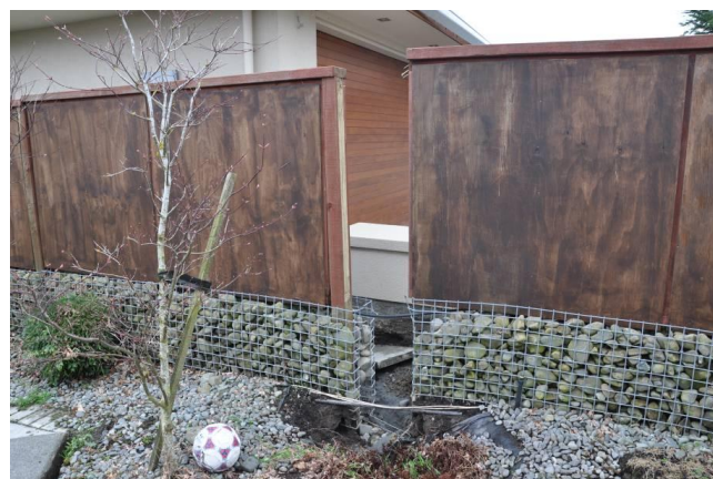
Figure 5.48: Separated fence line due to propagating ground fissure meandering between homes along Riverside Lane.
