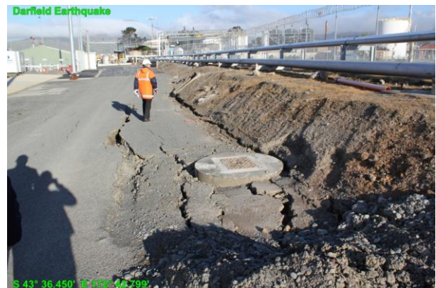
Figure 7.37: Settlement and lateral deformation at fuel transfer facility (43.60750°S, 172.71332°E).
