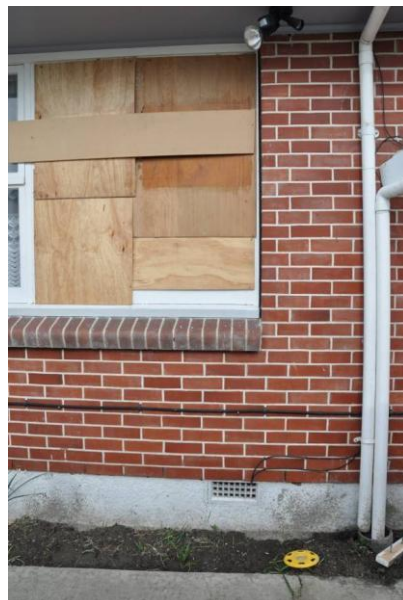
Figure 5.16: Residence along Charles Street (same structure as Figure 5.16). Damage to glass windows and between window and wall.
