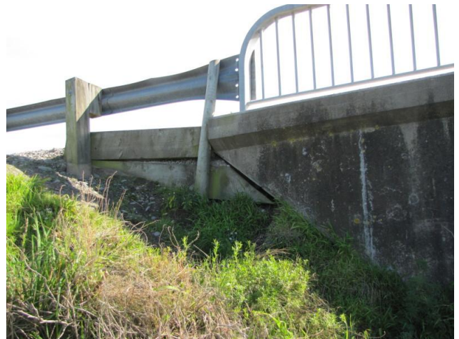
Figure 7.9: Back rotation of west abutment, Bridge Street Bridge.
