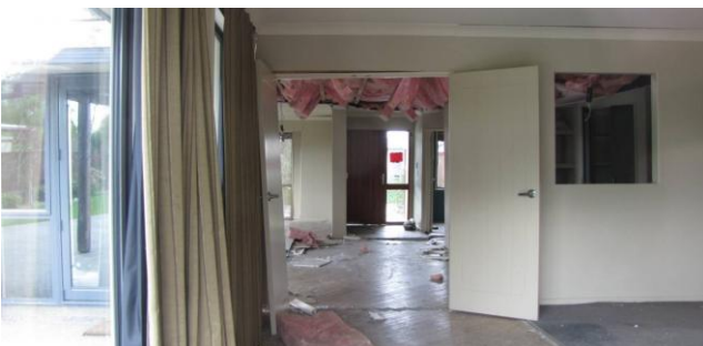
Figure 5.45: Interior view of residence at Riverside Lane. Note the two floor breaks visible in the picture
