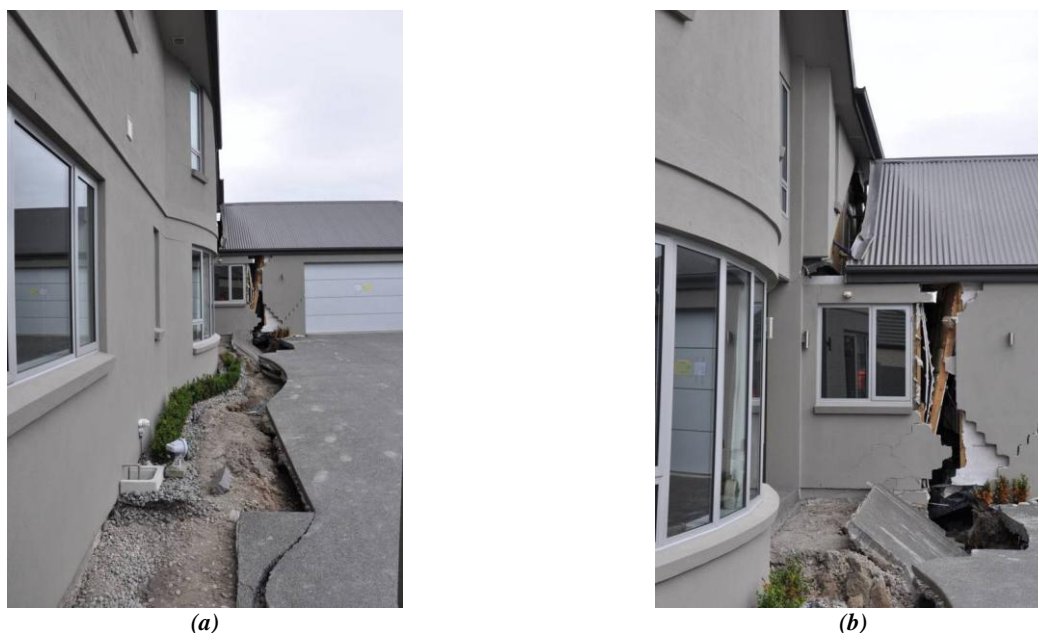
Figure 5.24: Damage to a residence along Courtenay Drive in the South Kaipoi residential community. Front entry articulates extensive damage as large ground spreading subtends into the superstructure.
