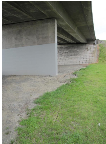
Figure 7.24: Evidence of liquefaction beneath Chaney's Overpass.
