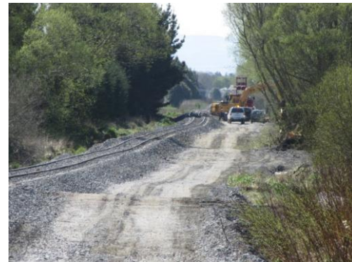
Figure 4.33: Damage to train tracks due to ground movement (position 3; 43.4068°S, 172.6489°E).
