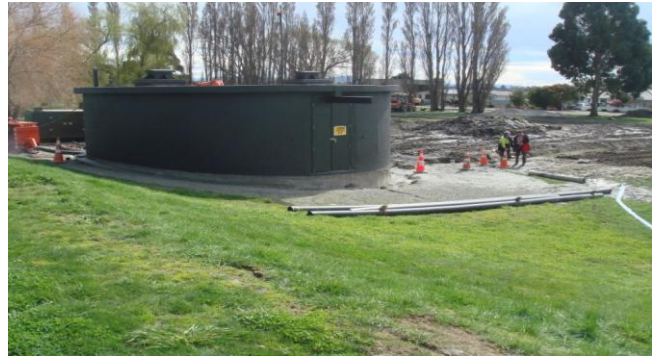
Figure 6.21: Photo 22: Settlement of tank structure. The locations of these photographs are denoted in Figure 6.2. (43.386918°S, 172.664412°E).
