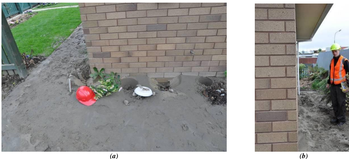
Figure 5.18: Red tagged residence on Charles Street. Extensive surrounding ejecta at perimeter of home.
