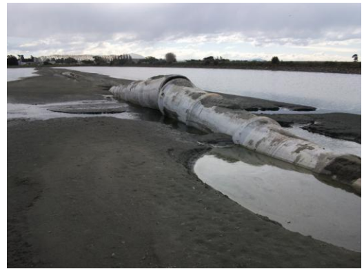
Figure 6.32: Buckled pipe protruding from Pond 1 during pond dewatering, and after pond level was lowered. Pipeline crown was at the pond invert prior to the earthquake. (-43.530867°, 172.705190°).
