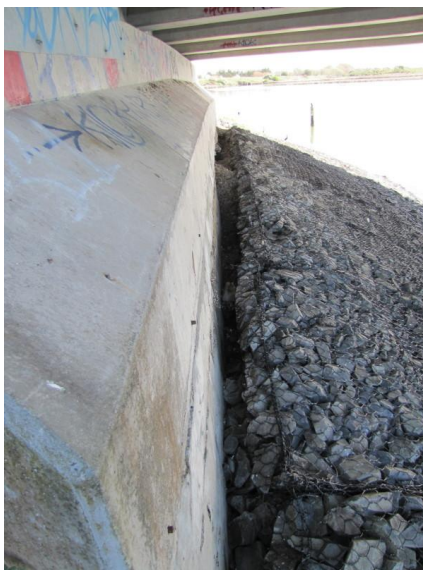
Figure 7.8: Gap between west abutment backwall and end embankment, Bridge Street Bridge.
