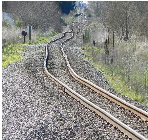
Figure 7.36: Damage to rail line at Woodford Glen (photo by L. Matthews and J. Overend).
