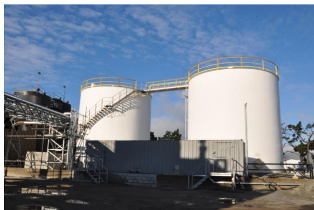
Figure 7.42 Tank 2 (right, large white tank) with Tanks 3 and 4 shown to the left (smaller grey tanks) at the Fulton Hogan Bitumen Plant. (43.6088°S, 172.7147°E).
