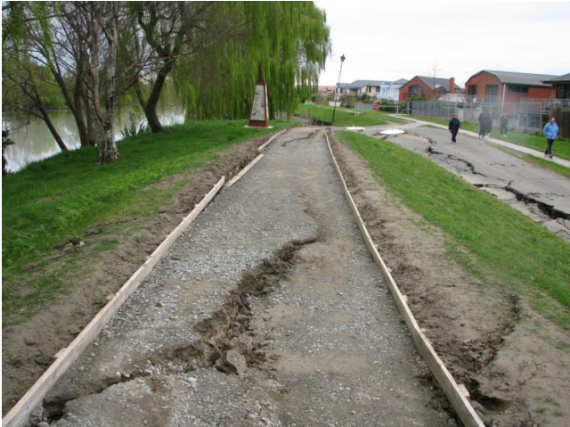
Figure 6.25: Photo 27: Lateral spread cracks along the top of the stopbank on the south side of the Kaiapoi River. The location of this photograph is denoted in Figure 6.2. (43.385693°S, 172.660688°E).
