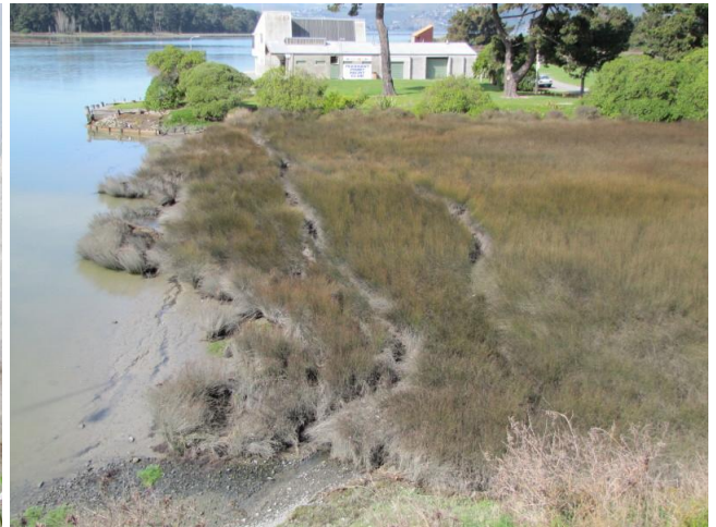
Figure 7.7: Lateral spreading on west bank, Bridge Street Bridge.
