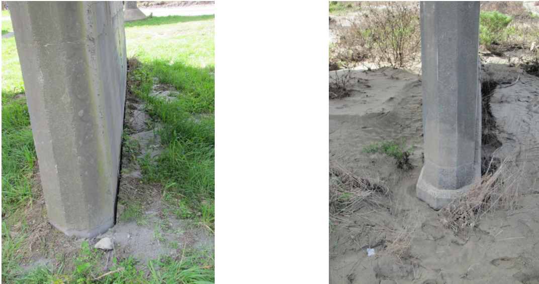
Figure 7.29: Evidence of liquefaction at Highway 1 bridge piers on the north side of the Waimakariri River.
