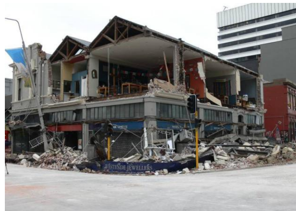
Figure 5.1: Structural collapse of a URM in the Christchurch Business District. (184 Manchester Street). Photograph courtesy of Assoc-Prof Jason Ingham.
