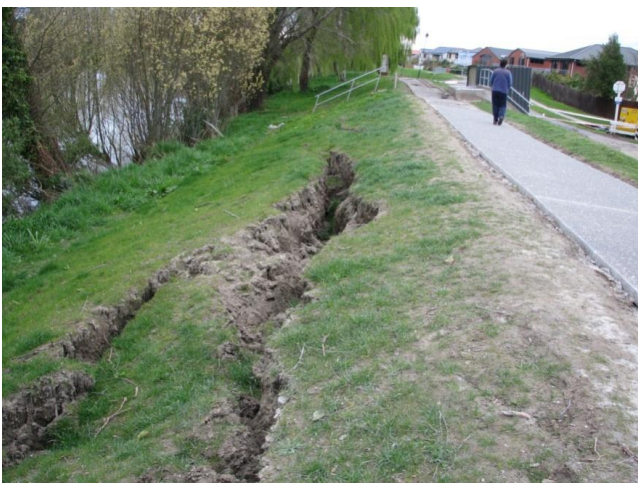
Figure 6.23: Photo 25: Lateral spread cracks along riverside stopbank on the south side of the Kaiapoi River. The location of this photograph is denoted in Figure 6.2. (43.385254°S, 172.660131°E).
