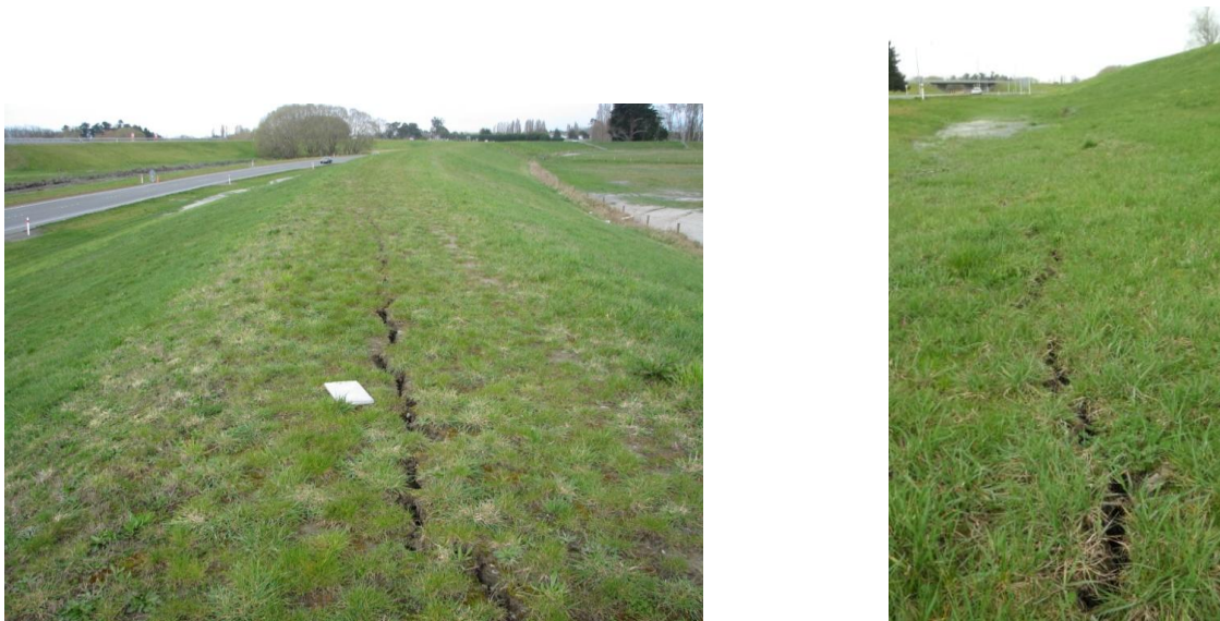
Figure 6.15: Photos 9 and 10: ~50 mm wide longitudinal cracks running along the crest (left) and base (right) of a secondary stopbank for the Waimakariri River. Photo taken looking southwest; SH1 on left of stopbank (43.430108°S, 172.643434°E).
