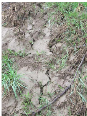
Figure 4.37: Ground damage adjacent to the bank of the Selwyn tributary near the end of Gillanders Rd (Darfield side). (Position marked as Photo 1 in Fig. 4.36).
