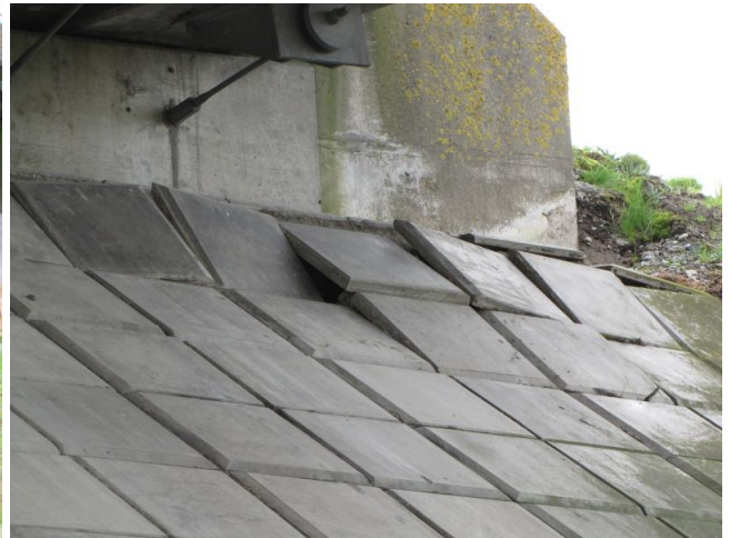
Figure 7.23: Displaced concrete tiles on end embankment for north abutment, Chaney's Overpass.
