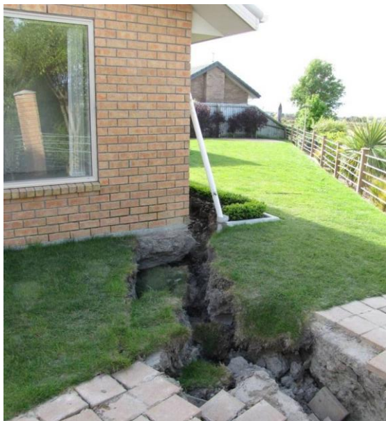
Figure 5.38: Lateral spreading compromising ground support beneath the concrete slab-on-grade house foundation. (Kokopu Street).
