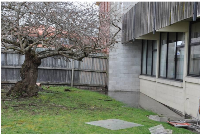
Figure 5.8: Property and Family Law Offices in Kaiapoi business district. (Williams St). View looking at west short axis end of the building.
