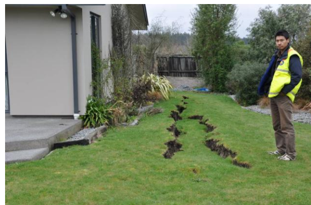
Figure 5.46: Lateral spread adjacent to residence at Riverside Lane. The location of this fissure is about 26 metres from the nearby Styx River.
