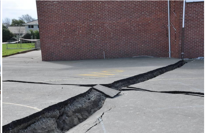
Figure 5.31: St. Paul's church in Dallington area - view looking north at ground failure, which continued through the building.
