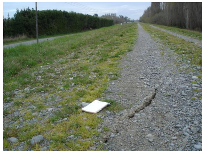
Figure 6.8: Photo 5: ~20 mm wide crack running lengthwise along the top of the stopbank on Coutts Island Rd. This crack was at the edge of the ~0.5 km stretch of the stopbank where significant liquefaction was observed. Photo taken looking southwest (43.423440°S, 172.632349°E).
