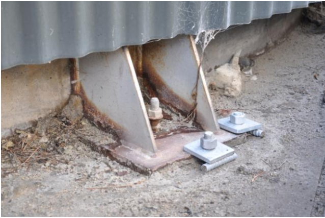
Figure 7.43: Typical repair to Tank 3 and 4 (addition of clamp plates). Note the pullout of the original anchorage. Fulton Hogan Bitumen Plant. (43.6085°S, 172.7149°E).
