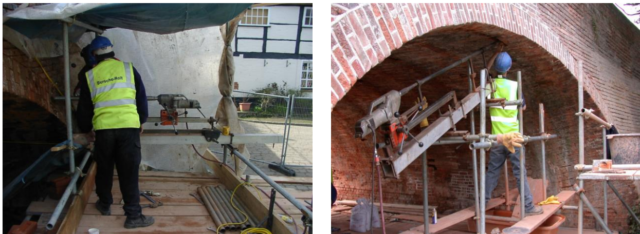
Figure 6. Drilling the transverse holes (left) and longitudinal holes (right) in the arch barrel
