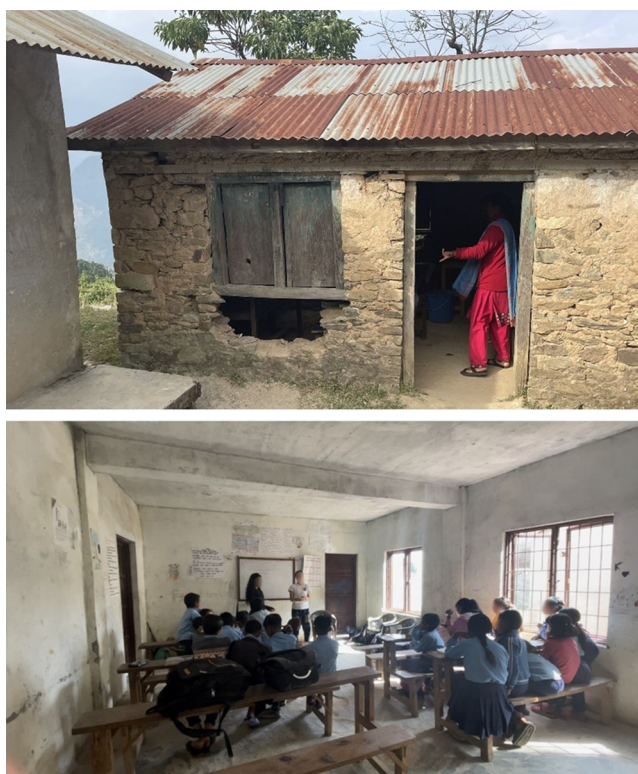
Fig. 1. School buildings and a classroom in Okhaldhunga, Nepal. Upper panel shows external wall of a school building that is crumbling and has a large hole under the window. Classrooms were often not watertight, with holes in the roof and walls. Gaps in the walls also meant sound travelled between classrooms and disrupted classes and student concentration. The lower panel shows the inside of a classroom. Wooden benches and a whiteboard were commonly the only materials available for students and teachers with very limited access to textbooks or other resources.
