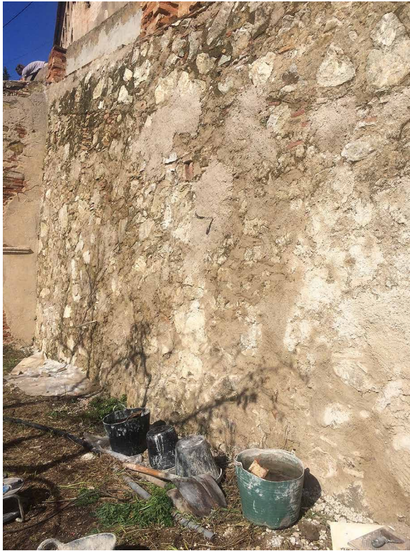
Figure 2 Uneven repair in Can Masdeu. (Source: Elisa Schramm.)
