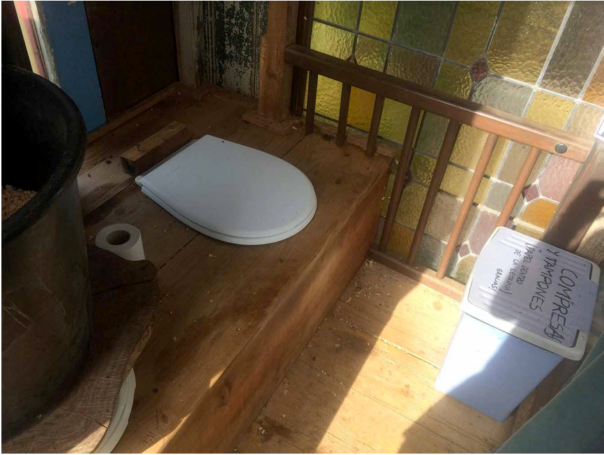
Figure 3 Inside one of Can Masdeu's compost toilets. (Source: Elisa Schramm.)
