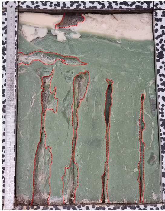
Fig. 28. Adhesive voids (highlighted with a red dashed line) in the interface between the filling foam and the skin layup.
