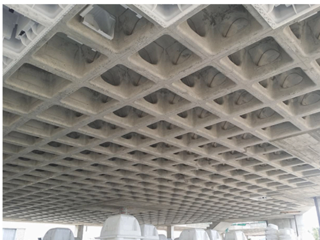
Fig. 3. Holedeck reinforced concrete floor system H0-45, with perforated beams to facilitate MEP services integration (image: HOLEDECK).
