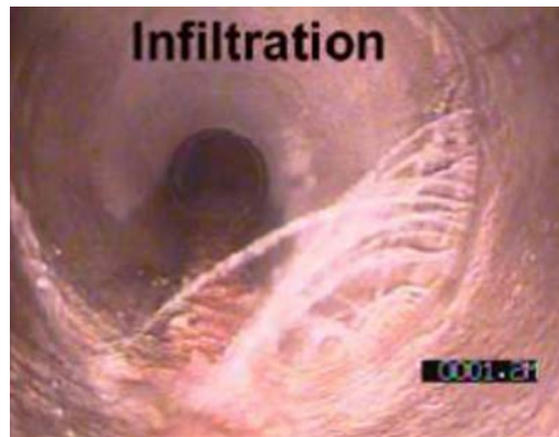
Figure 4.13 Example of clearly observable infiltration.
