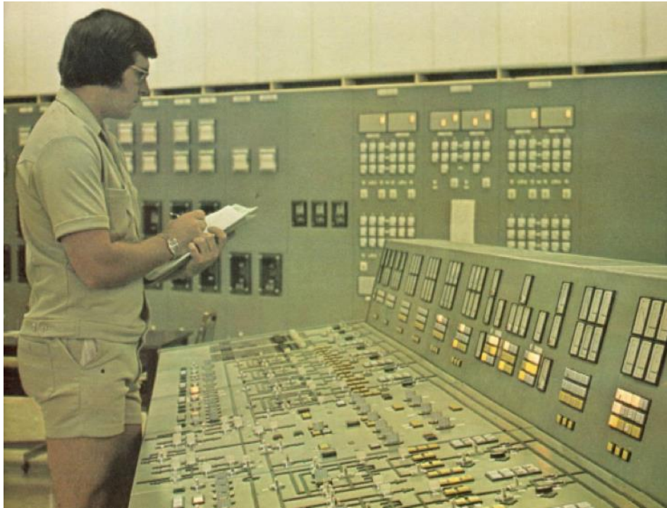
Figure 4 Eskom employee in centralized control center.
