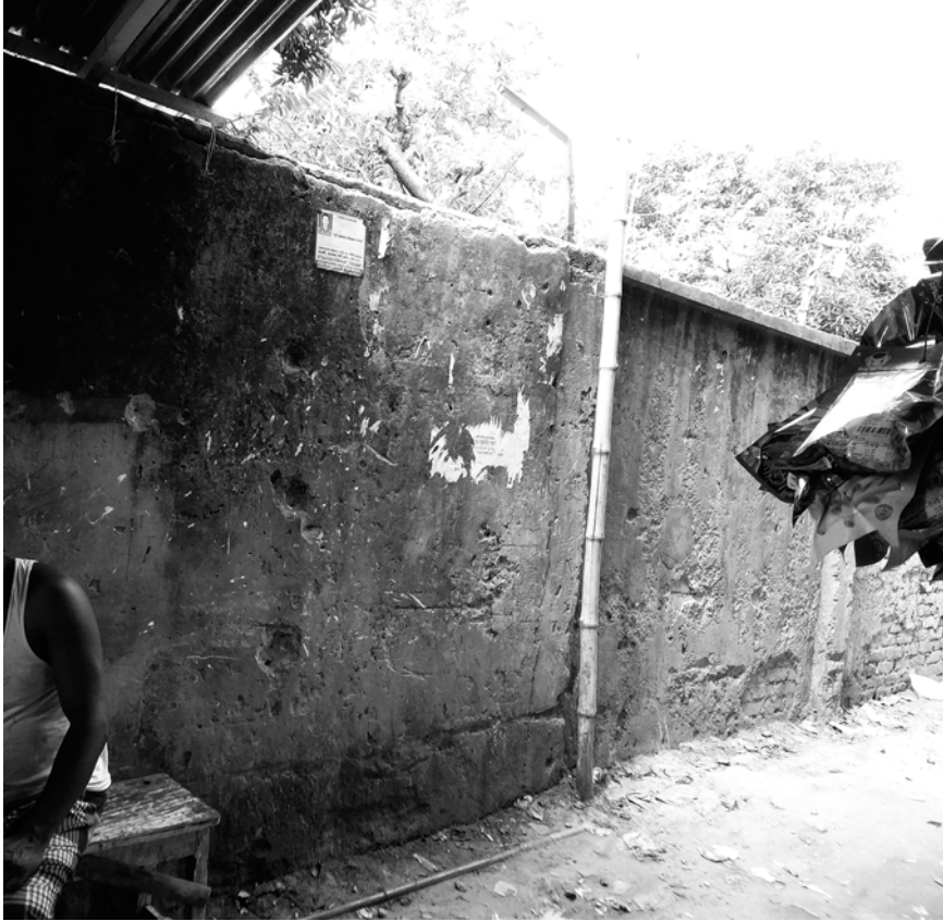
Figure 6 The wall was built with double the original thickness in this particular spot.
