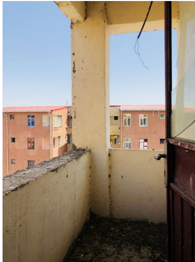
Figure 5. An unfinished balcony in a condo unit in Tulu Dimtu.
