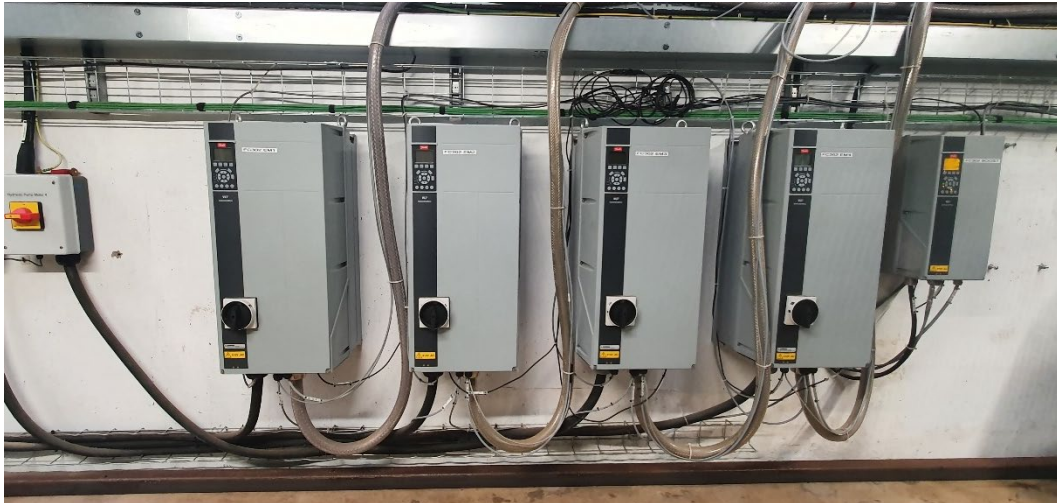
Figure 4. The VLT units controlling the power supplied to the electric motors. The four bigger units supply power to the motors driving the DDPMs, while the smaller VLT to the right controls the motor driving the pump feeding LP oil.
