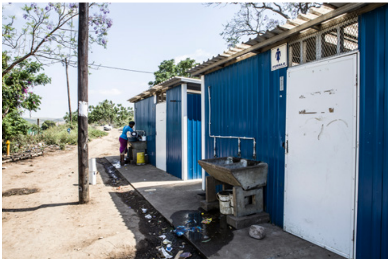
Figure 9.2 State provision of ablution facilities, Canelands and Coniston, northern eThekweni (source: Mark Lewis)
