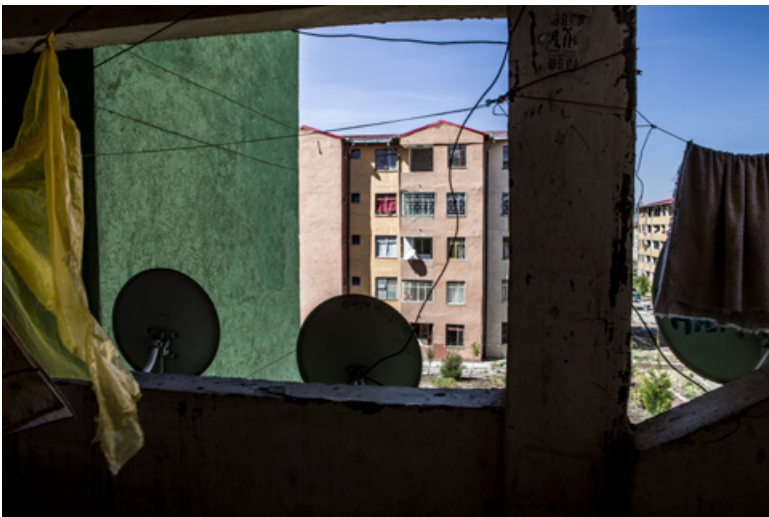
Figure 5.2 View from interior of Tulu Dimtu condominium housing showing incomplete construction (source: Mark Lewis)
