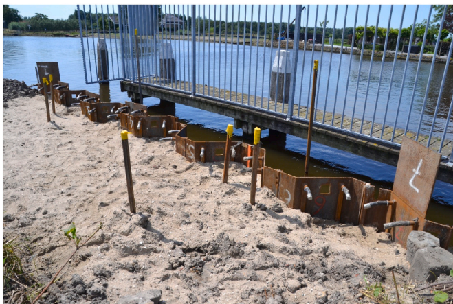
Fig. 7. Energy quay wall sheet pile installation. Heat exchanger pipes are observed above the ground surface attached to the sheet piles ready to be connected. Vertical pipes are part of the instrumentation system.
