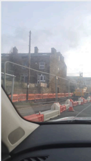
Can't cycle here as the road works make you closer to the cars. Very off putting (H8/GEN Y/FM)
