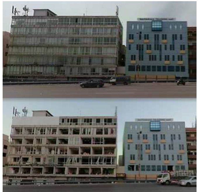
Figure 6 Different damage observed for different glazing systems at Location 2; before [top] and after [bottom] the explosion [3]
