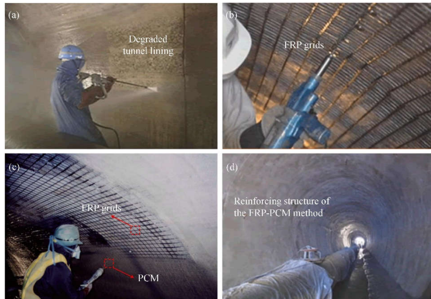
1 2 Fig. 38. Application of the FRP-PCM method on tunnel linings: (a) surface treatment; 3 (b) fix the FRP grids; (c) spray the PCM; (d) after the construction [161]. 4
