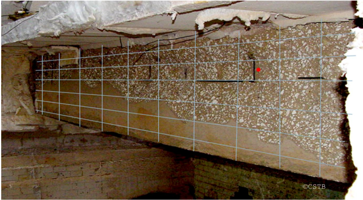
Figure 3: An example of grid for spalling depth distribution analysis on a rectangular beam
