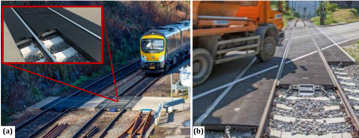
176 Fig. 7 Installation of rubber level crossing (a) in the UK (RosehillRail, 2022), (b) in Germany (STRAIL, 2022) 177
