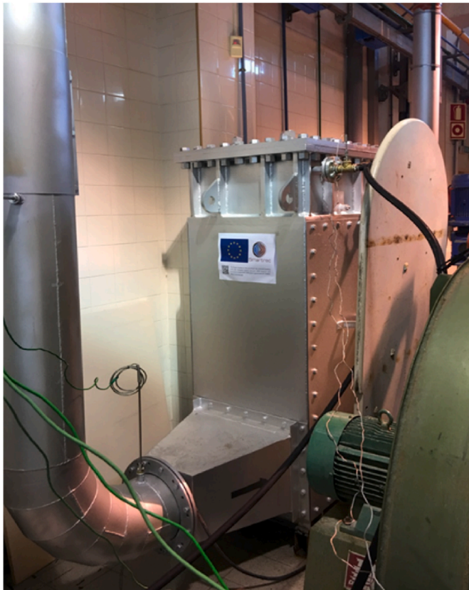
Fig. 4. Heat pipe heat exchanger retro-fitted to legacy ceramic furnace (courtesy of Hussam Jouhara, University of Brunel).
