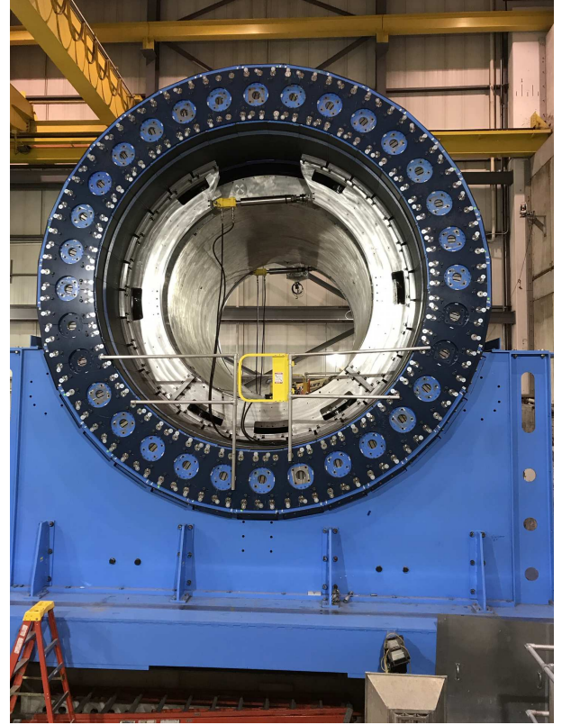
Figure 4: The BaBar solenoid in late February 2022, during installation in the sPHENIX experiment. The solenoid is surrounded by the barrel outer hadronic calorimeter and flux return. The barrel flux return (outer hadronic calorimeter) and BaBar solenoid are items planned to be reused by the ECCE experiment. The experimental cradle may also be reused.
