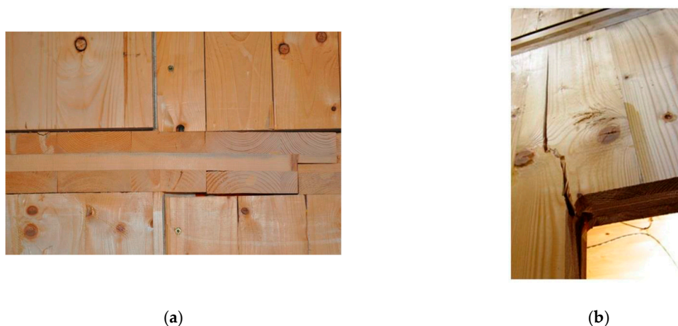
Figure 4. Timber panels damage observed in the quasi-static test of CLT buildings under large displacement: (a) embedment of wall panels into floor panels that causes the debonding of timber planks; (b) cracking in the corner of a large opening [19].
