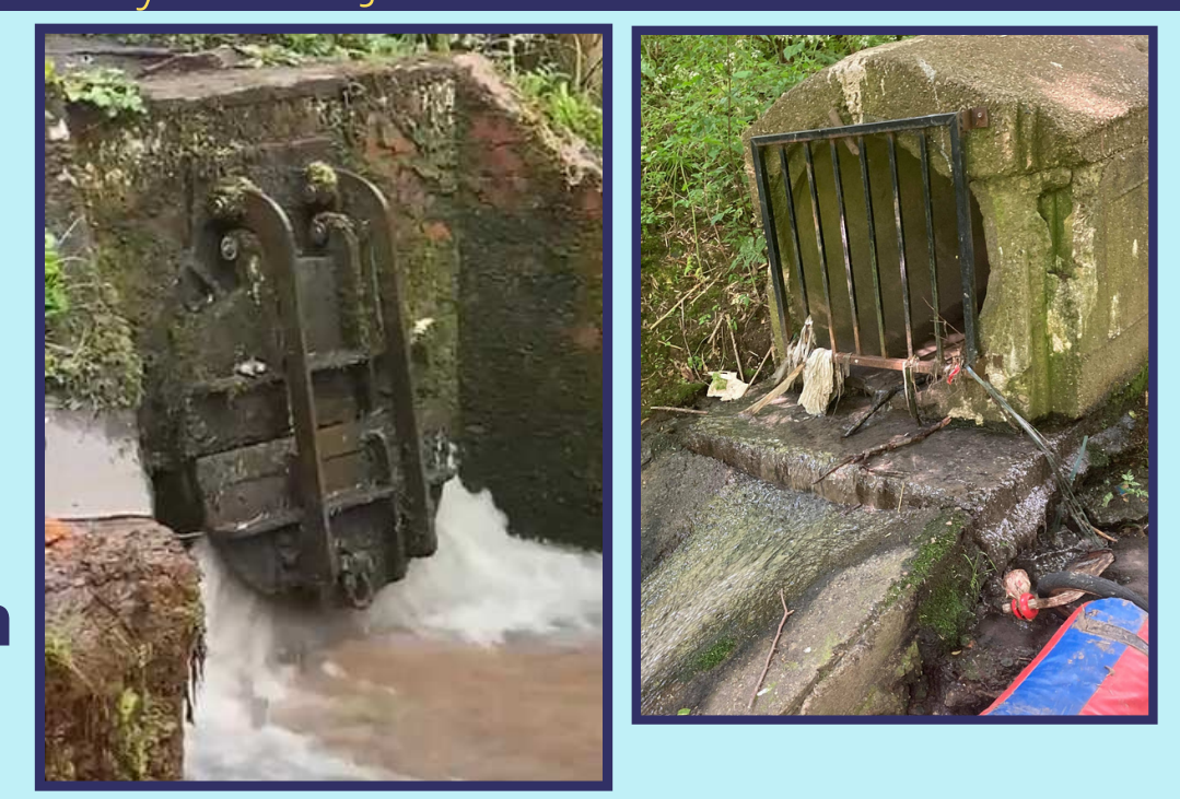
Figures 1 & 2. Combined sewer overflow outlets at two sample sites in Sheffield.
