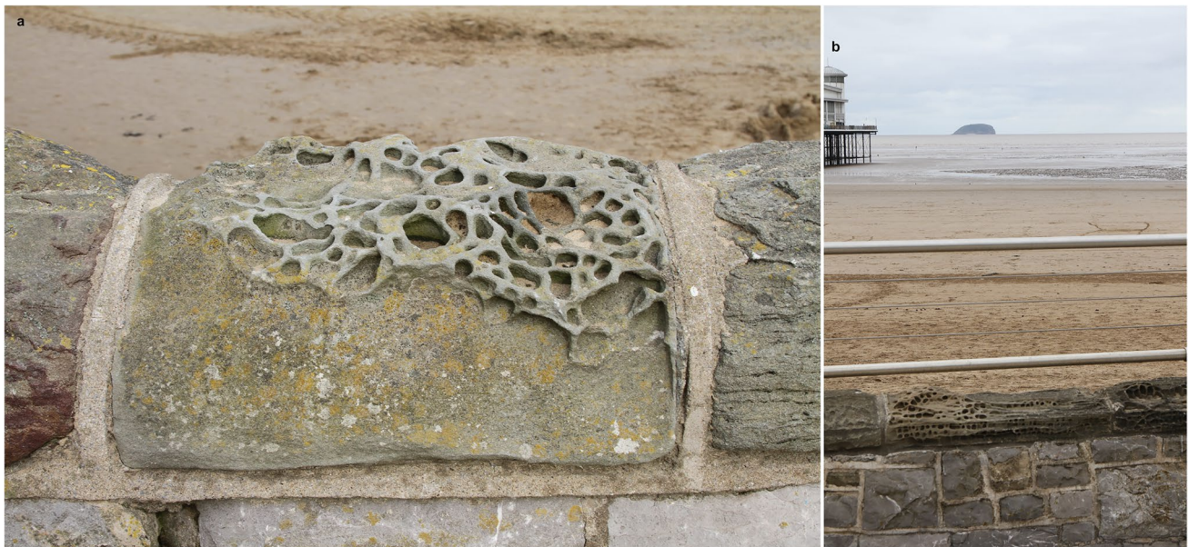
Fig. 5 a Coping stone of Forest of Dean sandstone differentially eroded by salt weathering to produce ‘honeycomb’ or ‘alveolar weathering’. Differences in the coping stone’s response to weathering can be seen left and right. b Honeycomb-weathered sandstone coping on the sea wall with recently (2016) added stainless steel rails. A por-
