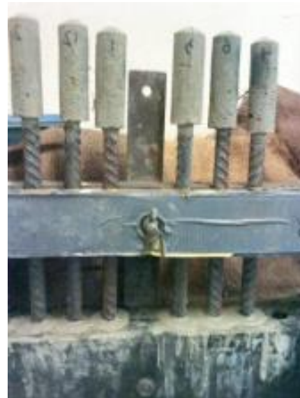
(d) Casting mortar on top of the self-amalgamating tape at the other end
