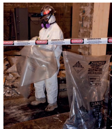
Fig. 2.7.6. An asbestos abatement worker uses appropriate personal protective clothing and equipment in the course of removing asbestos. Despite bans on the use of asbestos, the material may often be encountered in the course of demolition or rebuilding.
