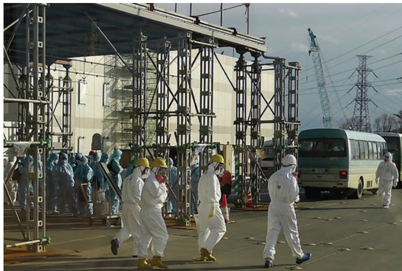
Fig. 5.15.2. More than two years after the accident at Fukushima Daiichi nuclear power plant, work continues to ensure that the damaged units remain stable. Here, workers in protective clothing and masks are shown outside the Emergency Response Centre, the main control hub at the site. Radiation exposure during childhood is the most clearly defined environmental factor associated with benign and malignant thyroid tumours.
