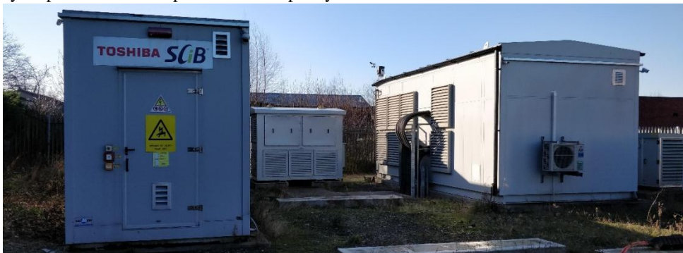
Fig. 3. Willenhall energy storage system
