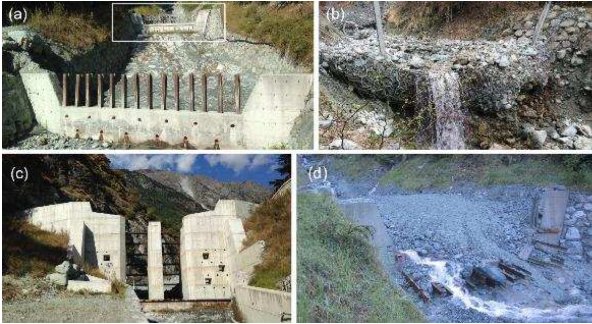
Fig. 2 The structural mitigation works along the Grand Valey torrent: (a) the two filter barriers at the Pèriere hamlet; (b) the steel net barriers; (c) the slit-filter barrier at Tromen; (d) the barrier at Pèriere (white rectangle in Fig. 2a) that collapsed in 2014. The position of each of these structures is indicated in Fig. 1 (photos courtesy of the Aosta Valley Autonomous Region).
