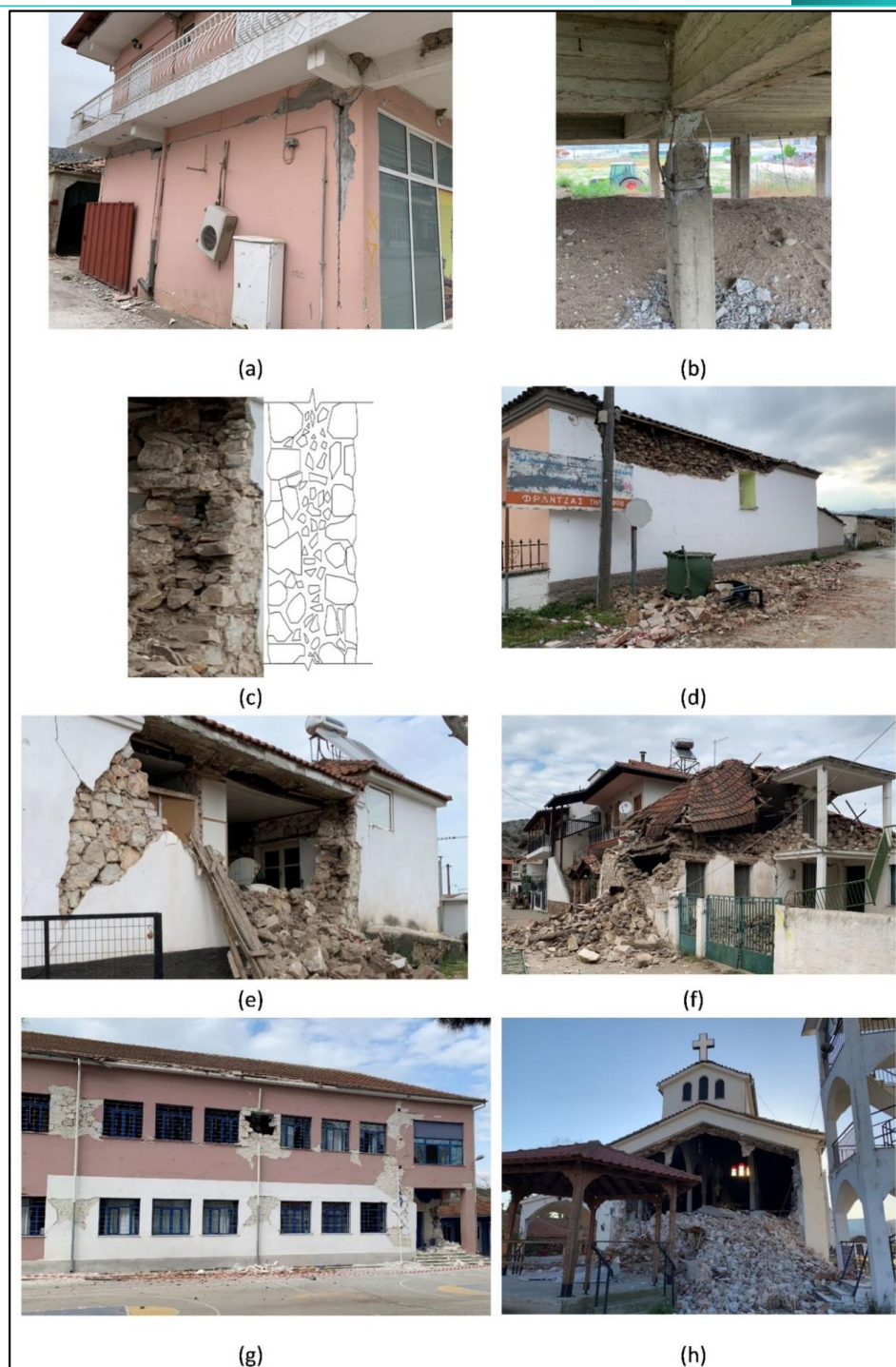
Fig. 13: a) Detachment of infill wall from RC frame in Damasi; b) Lack of proper detailing in an open ground floor in Damasi; c) Cross-section of a typical multi-leaf wall; d) Delamination of the outer leaf of the wall in a domestic building in Damasi; e) Out-of-plane collapse of masonry walls in Damasi; f) Out-of-plane collapse due to poor connection between the roof and masonry walls in Damasi; g) Damages in the School of Damasi; h) Out of plain failure of St Nickolas Church in Koutchochero.
