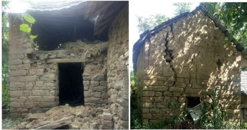
Fig 3: a Out of plane failure of wall, b development of cracks from openings
