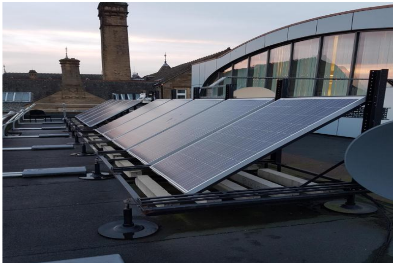
Fig. 1. Examined PV system installed at the University of Huddersfield, United Kingdom
