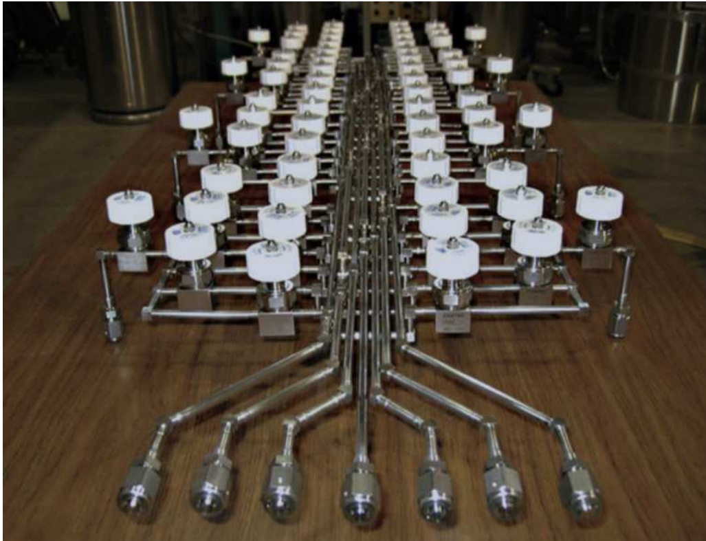
Figure 8.23. A gas analyzer switchyard that routes sample points to the different gas analyzers.
