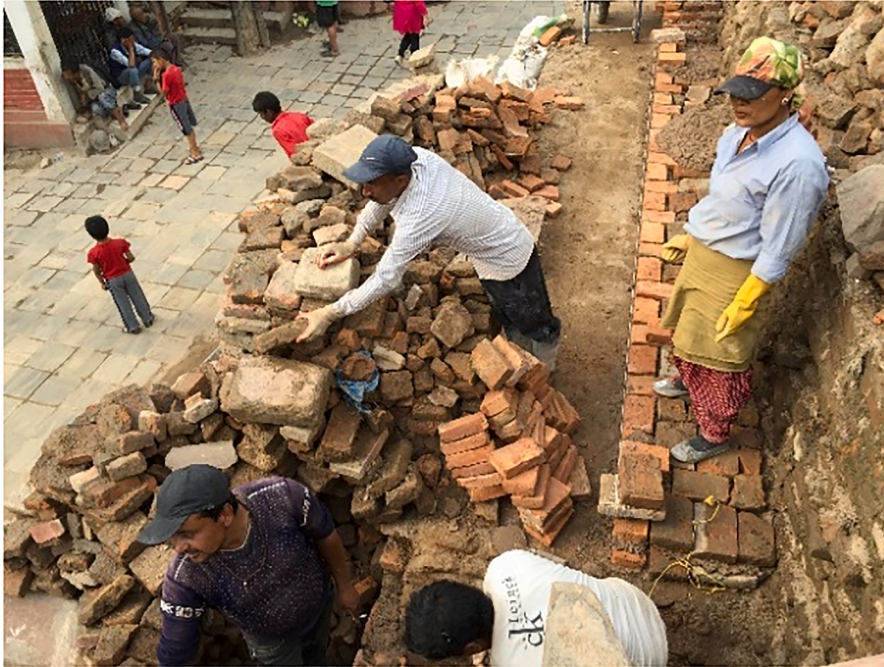
Fig. 5. A common intervention on the Nepalese temples is to remove the existing bricks in the perimeter of the plinth base and replace them with new material.
