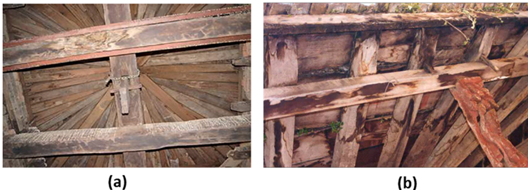
Fig. 2. (a) Timber floors poorly connected with limited bracing elements [48]. (b) Rotting roof beams and planks [46].
