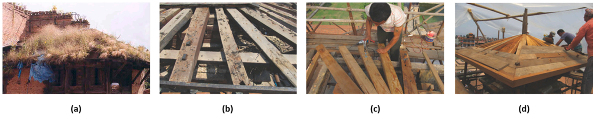
Fig. 4. (a) Vegetation attracted by the soil the soil layer existing in the tiers of the Nepalese temples [46]. (b) Rotten timber elements observed during inspections of the roofs of the Pagodas [51]. (c) and (d) Local material and techniques are used for the restoration of the roofs [51].
