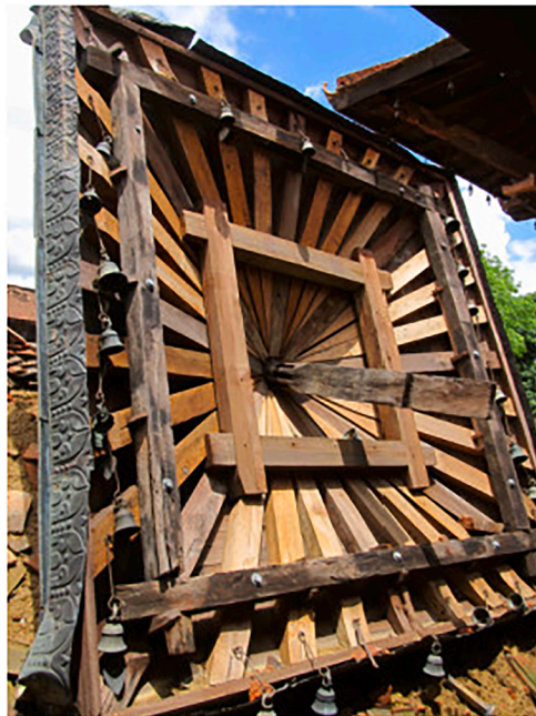
Fig. 21. The top tier roof of the South Taleju Tower toppled during the 2015 Gorkha earthquake [51].
