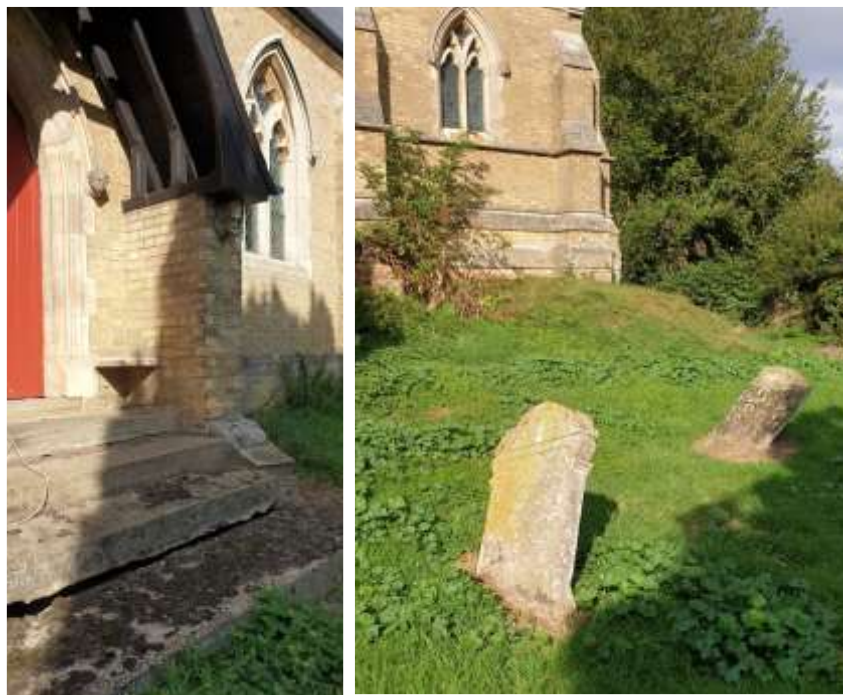
Figure 10: Subsiding steps at the Church entrance and collapsing gravestones in the churchyard at Ramsey St Mary's, Cambridgeshire. Built in 1859, the church was constructed on peat and soft clay using a foundation of wooden piles. It has remained relatively stable, although the spire had to be removed in 1920. By contrast, the surrounding land has subsided by several metres, leading to damage to churchyard monuments and necessitating the demolition of the Vicarage.
