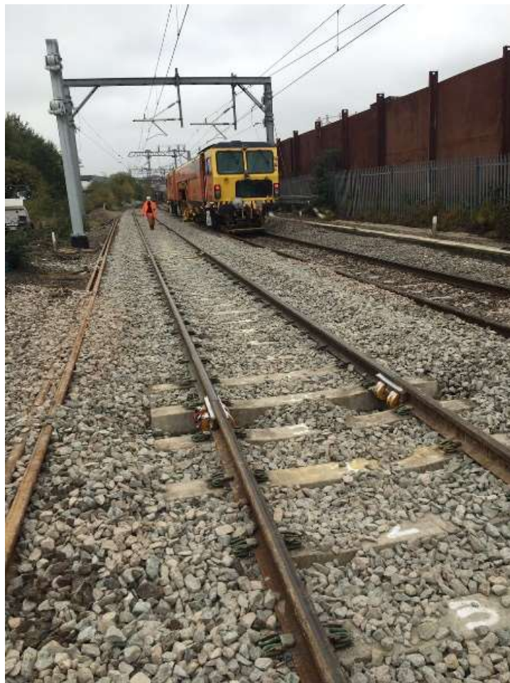
Figure 9: Tamping work on the railway track crossing Chat Moss. Over time, railway tracks settle with the passage of traffic; this is more likely to happen where the track passes over soft ground. The track may not settle evenly, resulting in track deformation. Tamping (i.e. packing - or tamping - the track ballast under the tracks) makes the tracks more durable, thereby ensuring good track alignment, smooth running and also preventing derailment.
