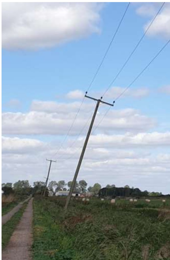
Figure 12: Subsidence damage to telegraph poles crossing drained peatland near Holme Fen, Cambridgeshire. (Photo – S. Page)
