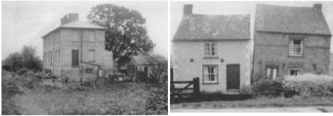
Figure 11: Images from Thompson (1957): Left - A house built on peat some 100 years previously with its foundations on clay. The peat level has subsequently been lowered by about 2 m by subsidence leaving the house entrances above ground level. Right - Two Fenland cottages leaning away from each other as a result of peat subsidence.
