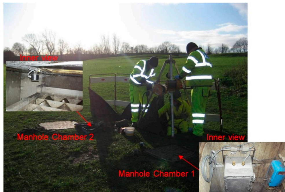
Figure 12. Practical implementation of the proposed acoustic system used in phase 2 field experiments.
