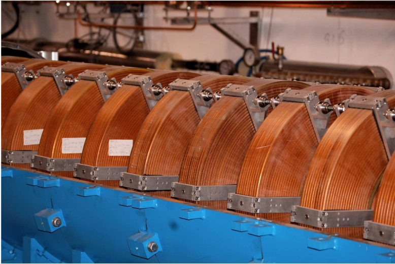
Fig. 12.3. Solenoid coils embedding the first accelerating S-band structure; the upper iron shield is removed.
