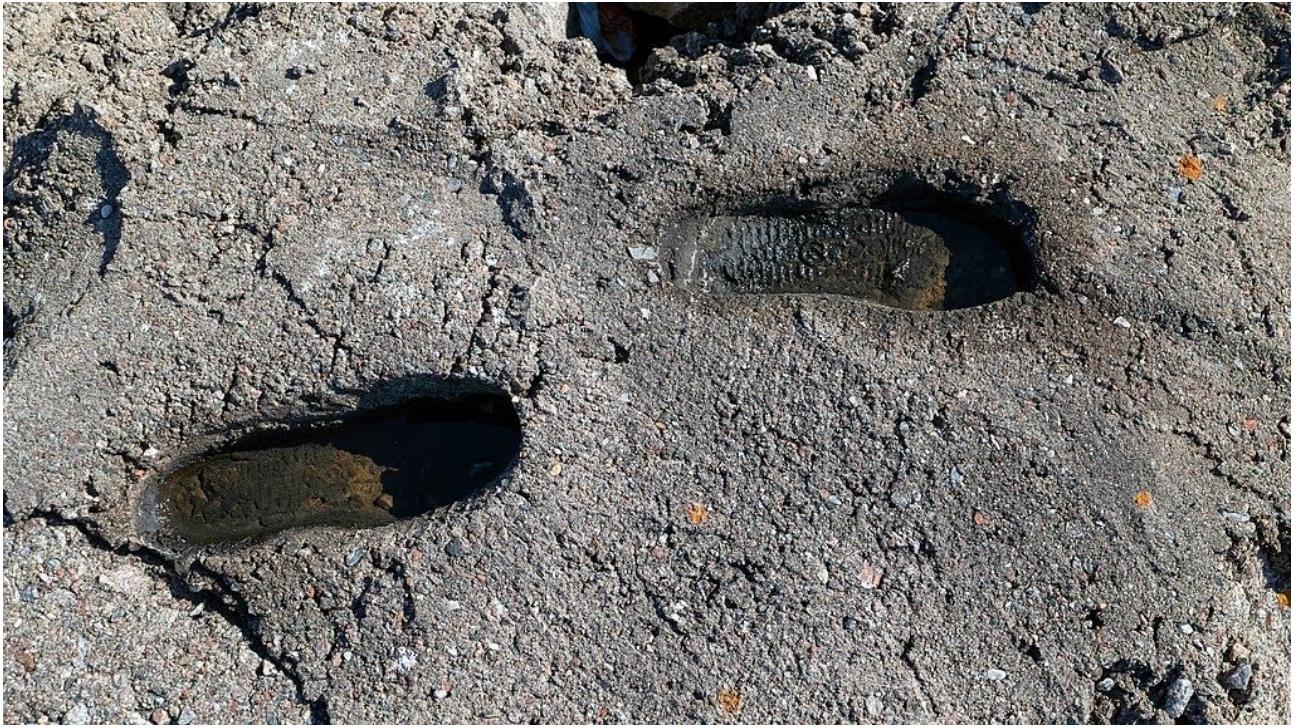
Figure 3: Footprints made by Ecco shoes in concrete on the old quay in Govik, Lysekil Municipality, Sweden. This file is made available under the Creative Commons CC0 1.0 Universal Public Domain Dedication.
