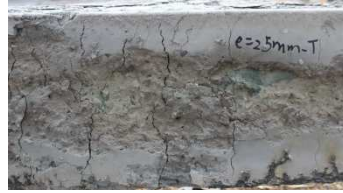
(c) Concrete cracks in tension zone (TRC-0.5-25)
