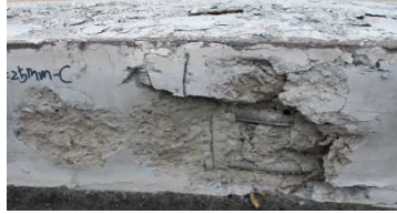
(b) Concrete crushing and re-bar buckling in compression zone (TRC-0.5-25)
