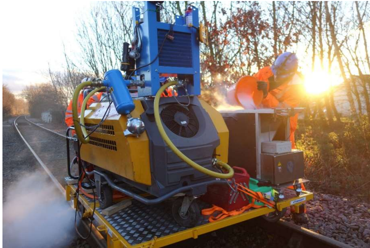
Figure 2. The track trolley mounted equipment in use on a low traffic freight line in South Yorkshire
