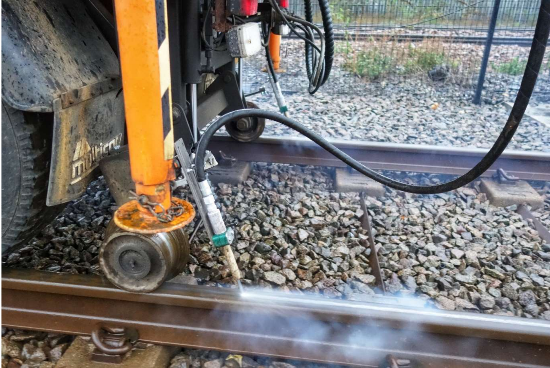
Figure 4. The Cryogenic Cleaning system mounted on the RRV Multicar at Sheffield Supertram Depot, cleaning heavily oxidised track
