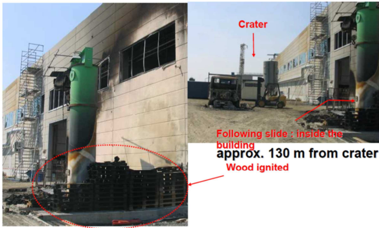
Fig. 10. Damage caused to wooden pallets 130 m from the crater [14].
