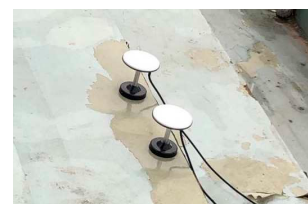
(c) Direct channel antenna.
