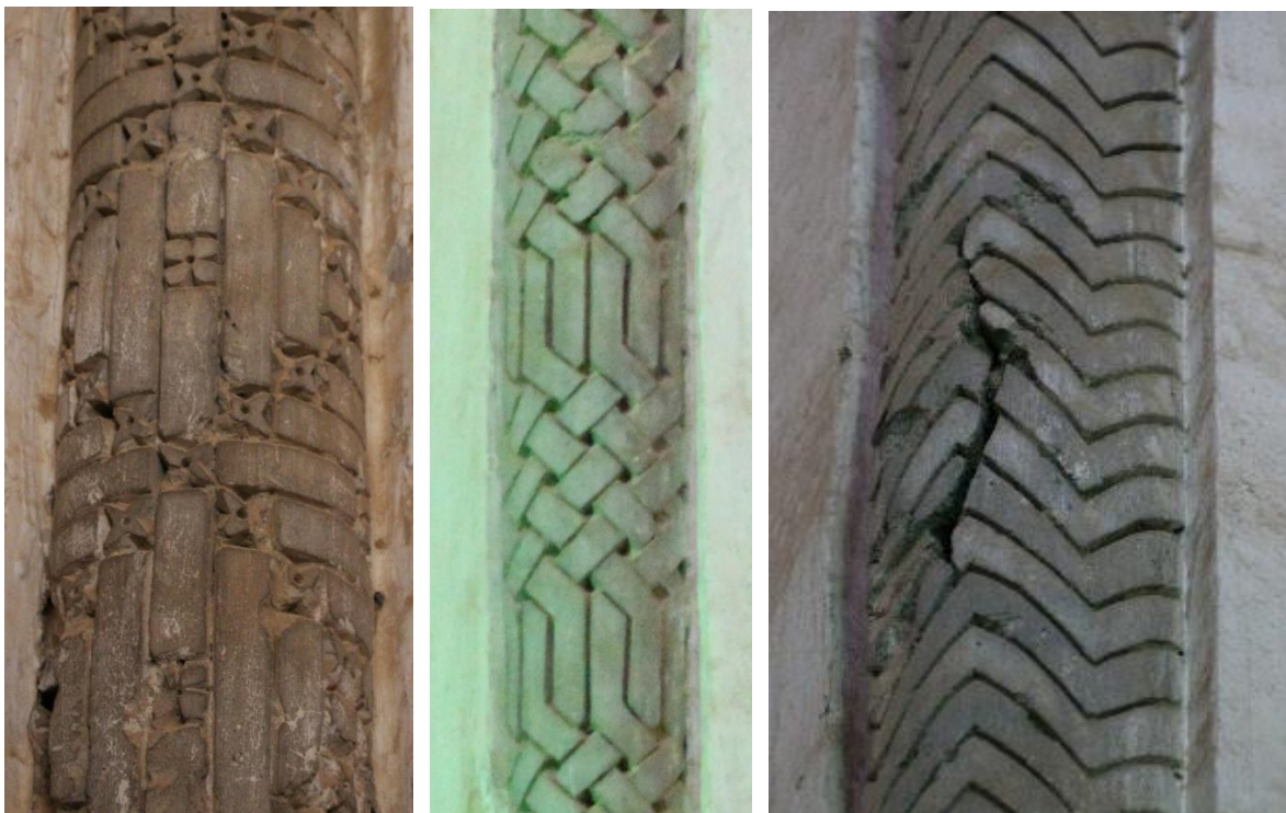
Figure 11: Engaged column details from the south (L), west, (C) and north (R) walls of the shrine
