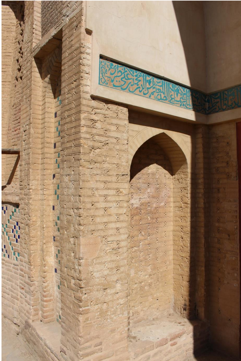
Figure 18: Incised mortar bed patterns in brickwork on left side of the entrance to the mosque and the shrine in Natanz
