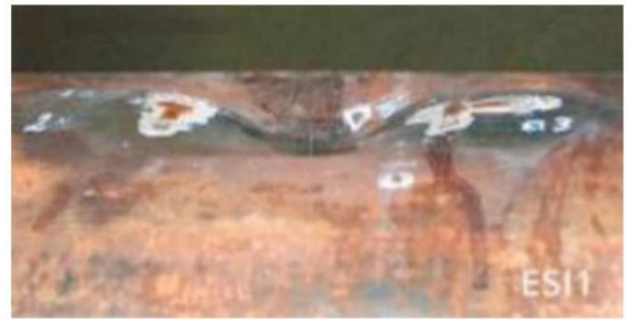
Figure 2. Dent in pipeline
