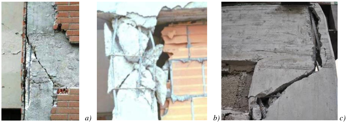
Figure 2. Local failures of RC frames due to the interaction with infills: a) Failure of a joint; b) Failure of a column end; c) Failure of column and joint.
