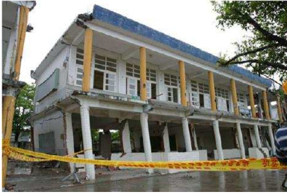
a) Final stage of a specimen from in-situ tests with URM walls
