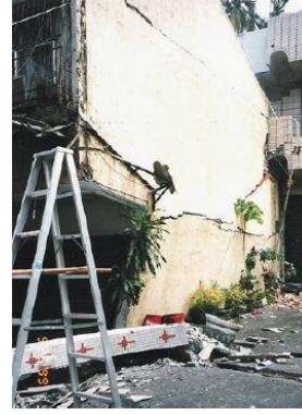
b) A confined masonry building during Chi-Chi Earthquake, 1999
